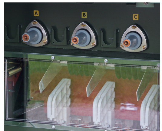
Confirming the visible break through the AIS windows eliminates the need to move the 600A connectors. Sufficient space is provided for feed-through bushings for parking of elbows on parking stands.
